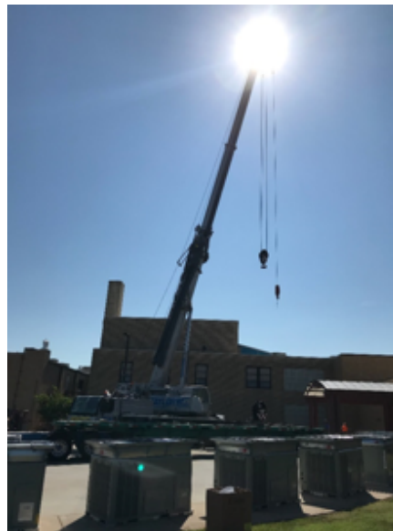
Nelson Bird in our Joplin office, captured the crane laying roof top HVAC Units
